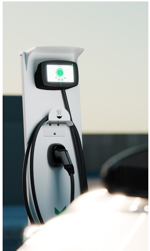
Wallbox Commander 2 on a pedestal in a commercial parking lot.
